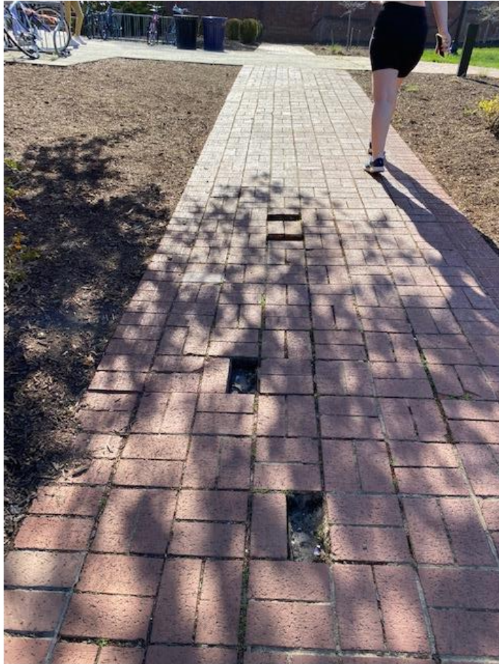
(this has a temporary repair, 4/14/23)
